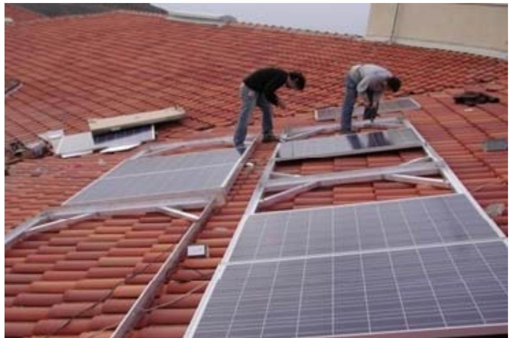
Solar Panel Installation in Bozca island, Turkey as Part of UNIDO-ICHET Hydrogen Island Project. Photo Courtesy of UNIDO-ICHET
